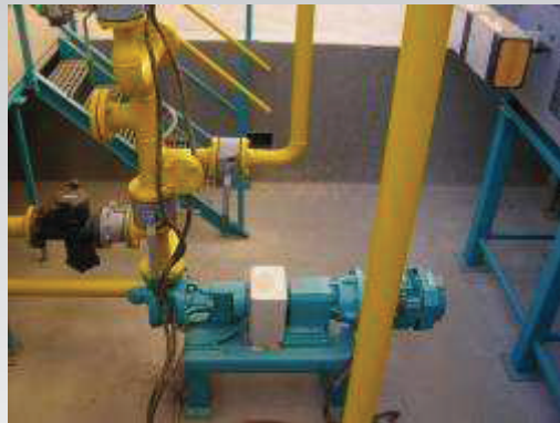
Bulk storage refilling pump
